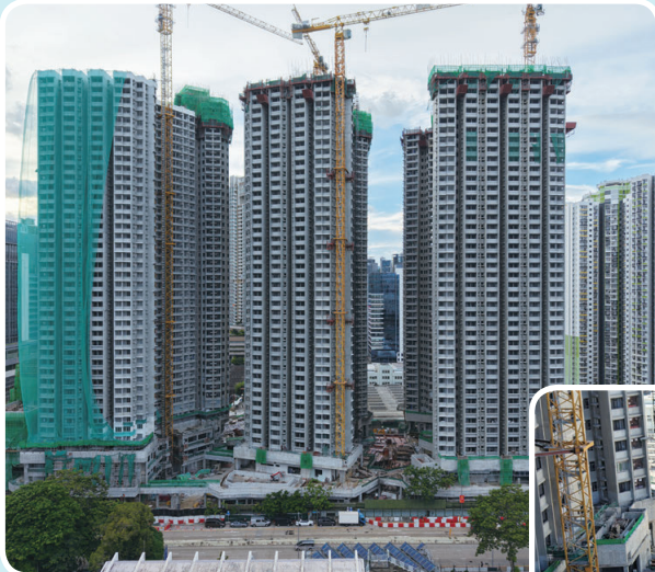
Construction of Public Housing Development at North West Kowloon Reclamation Site 1 (East)
