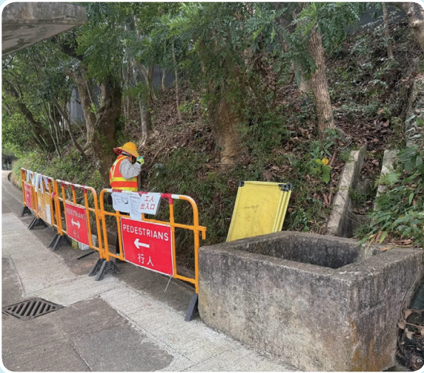
Description: Open channel cleaning work on Clear Water Bay Road 描述：清水灣路明渠清理工程
