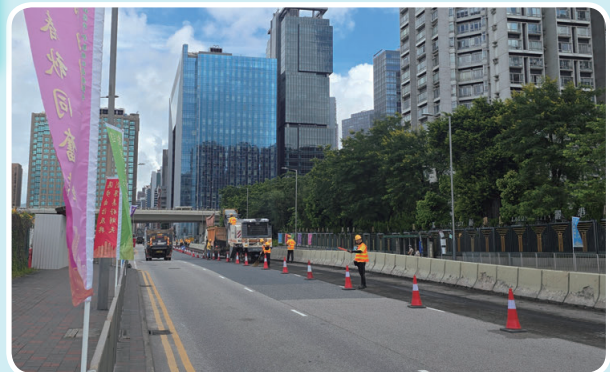
Description: Cold mill the existing bituminous road pavement for subsequent road resurfacing
